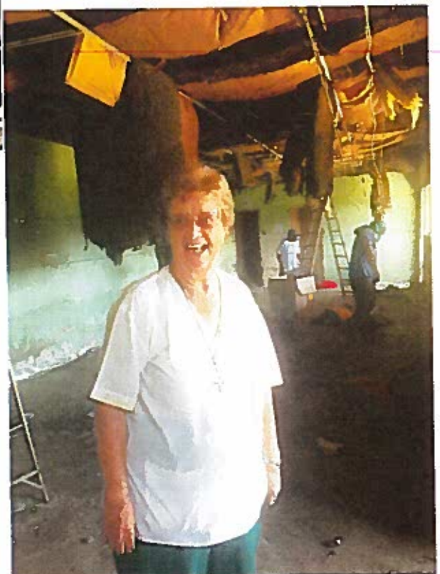
Sister Lillian Bockheim, OP as the demolition begins in her 49th year of service.
